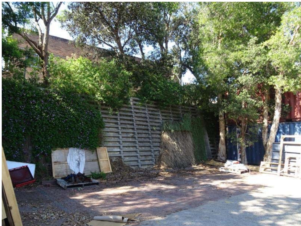
Figure 7: Retaining wall along the southern boundary of the site, indicating the significant level change between the site and McPherson Lane (approximately 4m)
